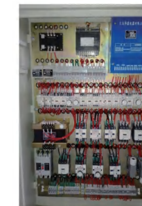
Slewing&Trolley Control Panel Box
